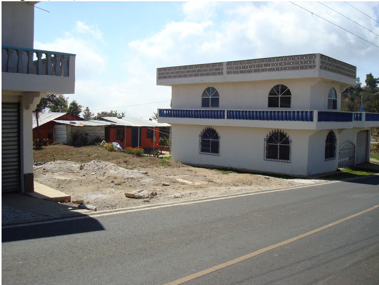
Figure 2. New home construction for an absentee migrant with his childhood home in background, Sinai, Guatemala.
